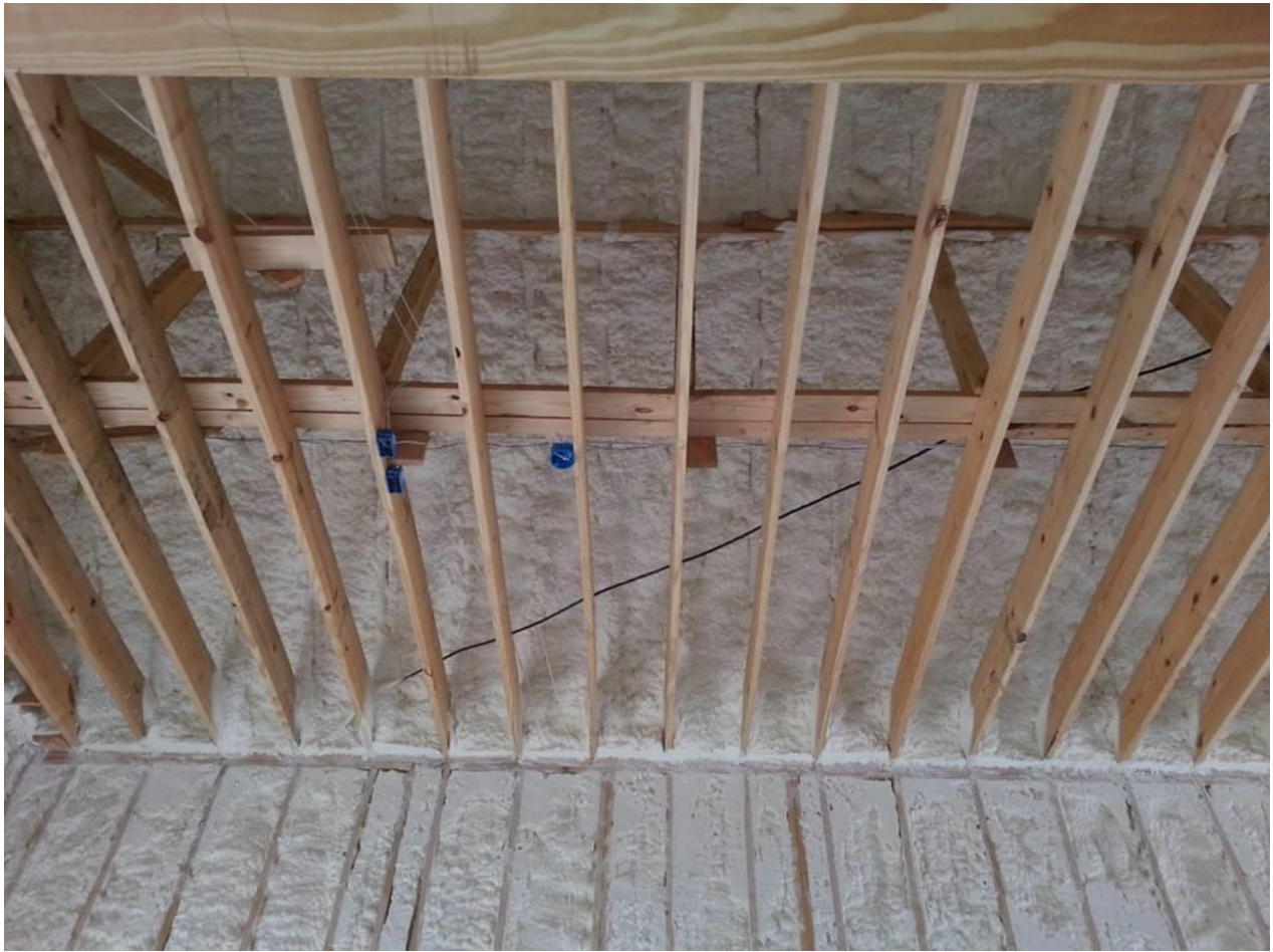
Figure 2: Looking upward through the open ceiling, if the exterior wall and roof deck assemblies both contain spray foam then a continuous insulation and airtight layer is established from the base of the walls to the peak of the roof. A very energy efficient enclosure results. Image Courtesy of D7 Spray Foam Insulation, Houston TX
